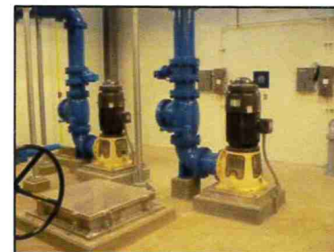
Supplemental Backwash Pumps
