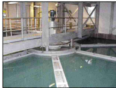
Solids Contact Clarifier
